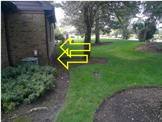
Grading / Drainage: Negative slope.
