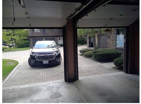
Overhead Garage Doors:
