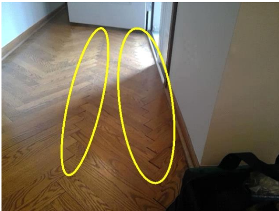
Entrance/Dining Room: Floor uneven and popping up.
