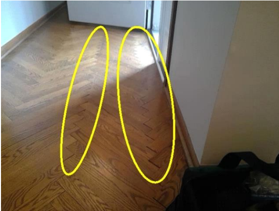
ENTRANCE/DINING ROOM: Floor uneven and popping up.
