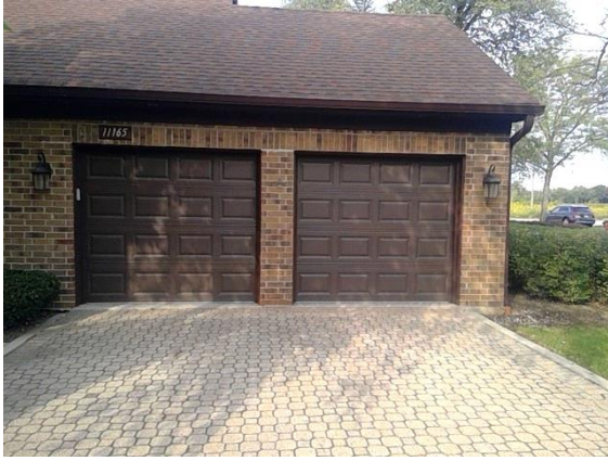
Overhead Garage Doors:
